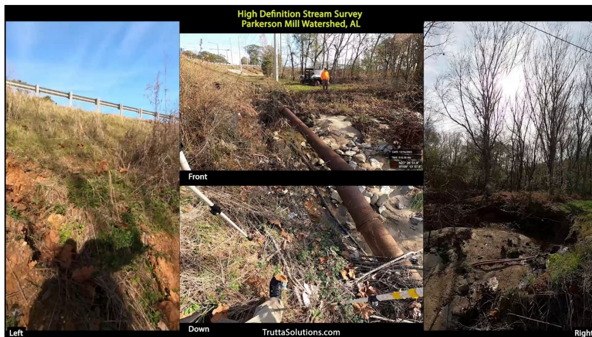
Figure 46: StreamView image of one of the worst reaches based on the Overall Condition score influenced by infrastructure (e.g., culverts and exposed pipes), along AU Beef Unit segment of the survey.
