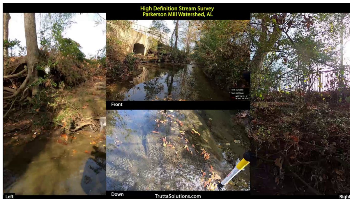
Figure 47: StreamView image of one of the worst reaches based on the Overall Condition score influenced by infrastructure (e.g., culvert), along the Coliseum segment of the survey.
