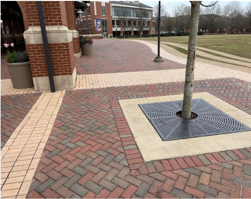
Permeable Pavers along Heisman Drive. (Heisman Drive - Tree & Landscape Improvements for Campus Green Transit Hub Area- AU Project # 20-384)
