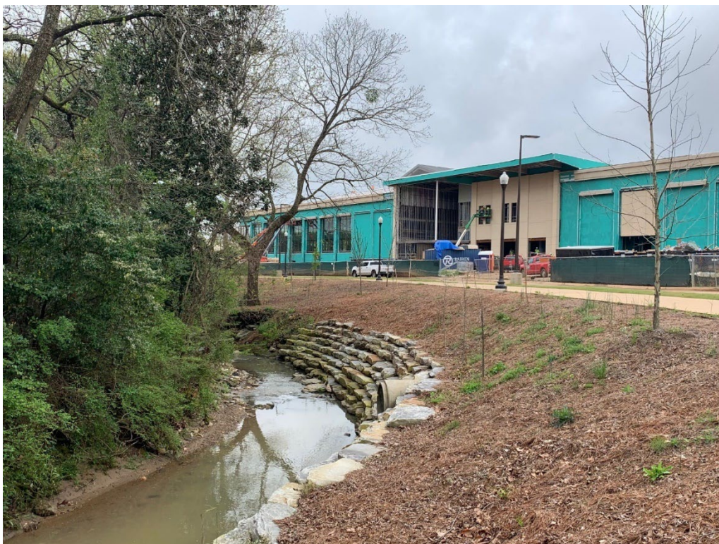
Stream Restoration along Biggio Drive adjacent to Parkerson Mill Creek Greenway (Football Performance Center - AU Project 19-441).
